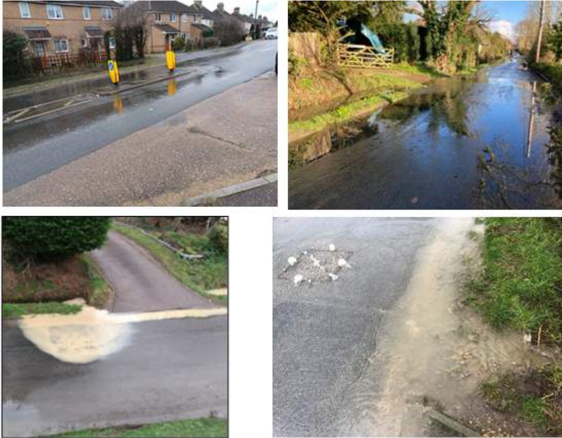
Figure 16. Photos demonstrating foul water flowing up through manhole covers on Swaynes Lane and Barton Road.
